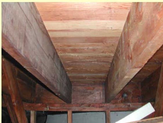
No insulation under original portion of House G
