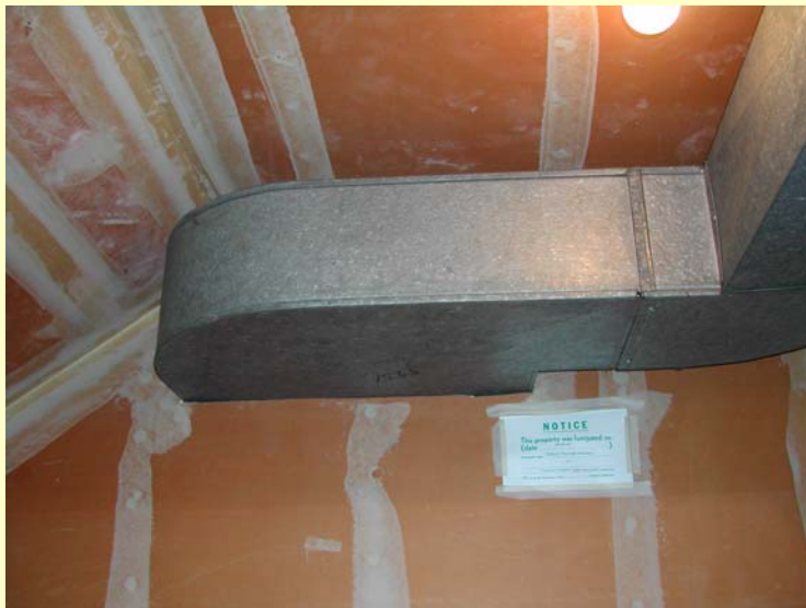
Uninsulated ducts in two PV homes
