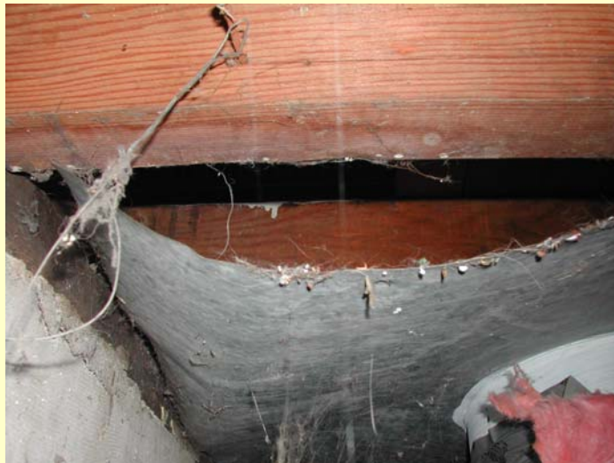
Gap in unducted return, Home G
