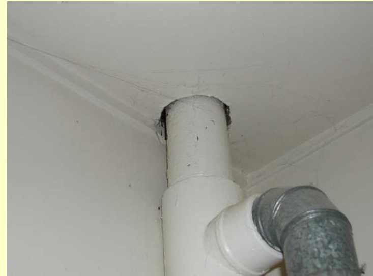
Unsealed ceiling penetration, House G
