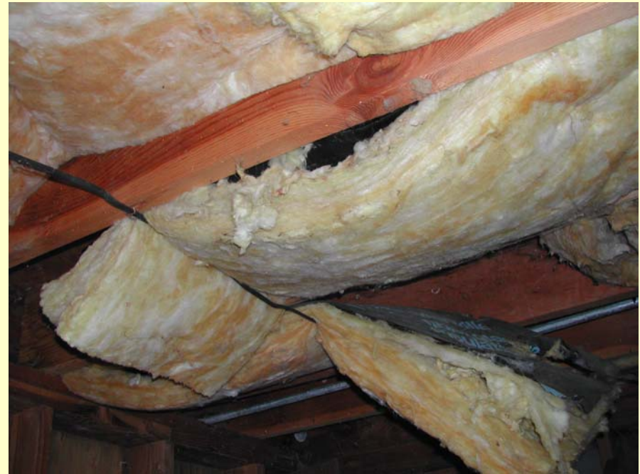
Fallen insulation under Portola Valley home
