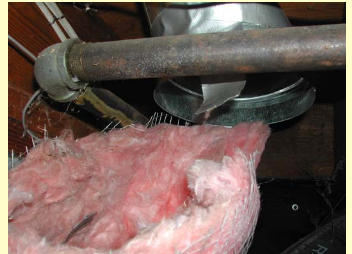
Disconnected duct, House G
