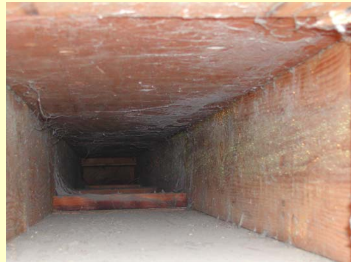
Extremely leaky unducted return, Home B
