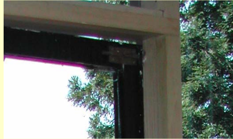
Large gap visible above door in Home D
