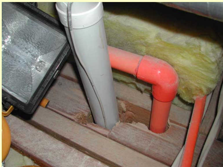
Unsealed plumbing penetrations, House F
