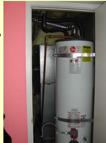
Utility closet in Home A
